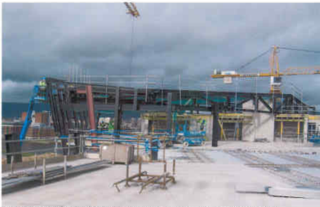
Photo 4: Hull 4 Roof Steel (Note: MBF in cherry picker working on cladding rails) (as at 8/9/10)
